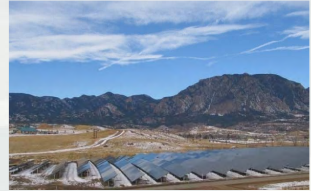
Fort Carson Photovoltaic Array
