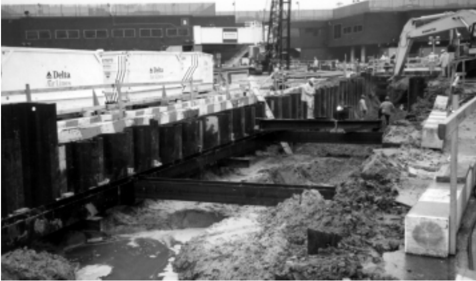
Emergency trench shoring design for new International Arrivals Terminal at JFK Airport.
